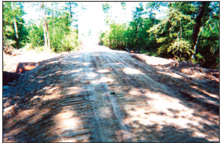
Culverts and road building are part of the BMP guidelines found in the Louisiana Recommended BMP manual.
