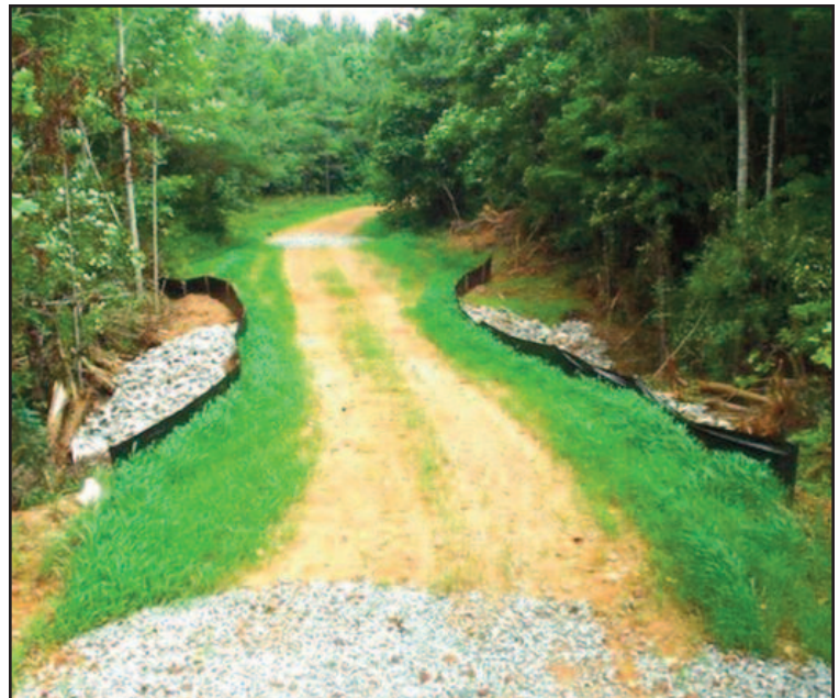
Corrective actions following harvesting activities protect your land from erosion and damage from log trucks.
